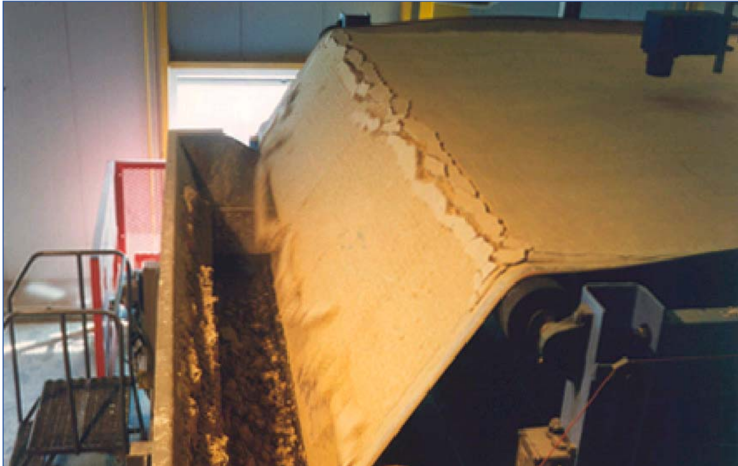
Wet LSFO FGD Gypsum Dewatering Filter
