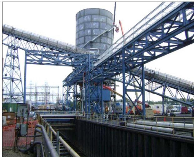
Pipe and Cable Tray Back to Byproduct Silo
