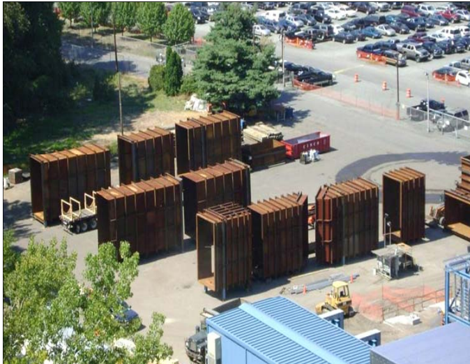
Ductwork in Staging Area
