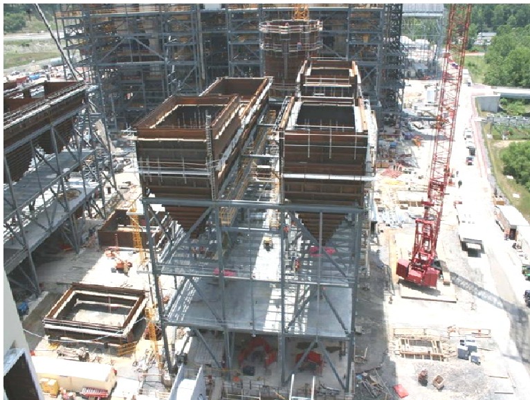
PJFF Installation with CDS
