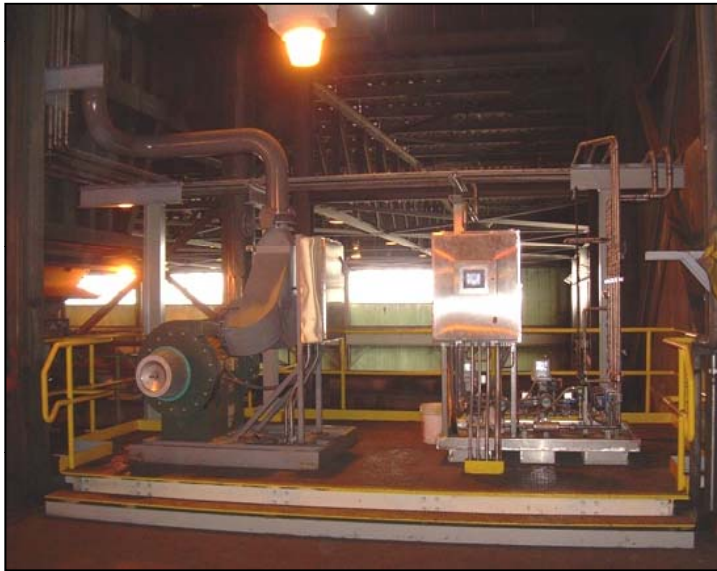
SNCR Permanent System
