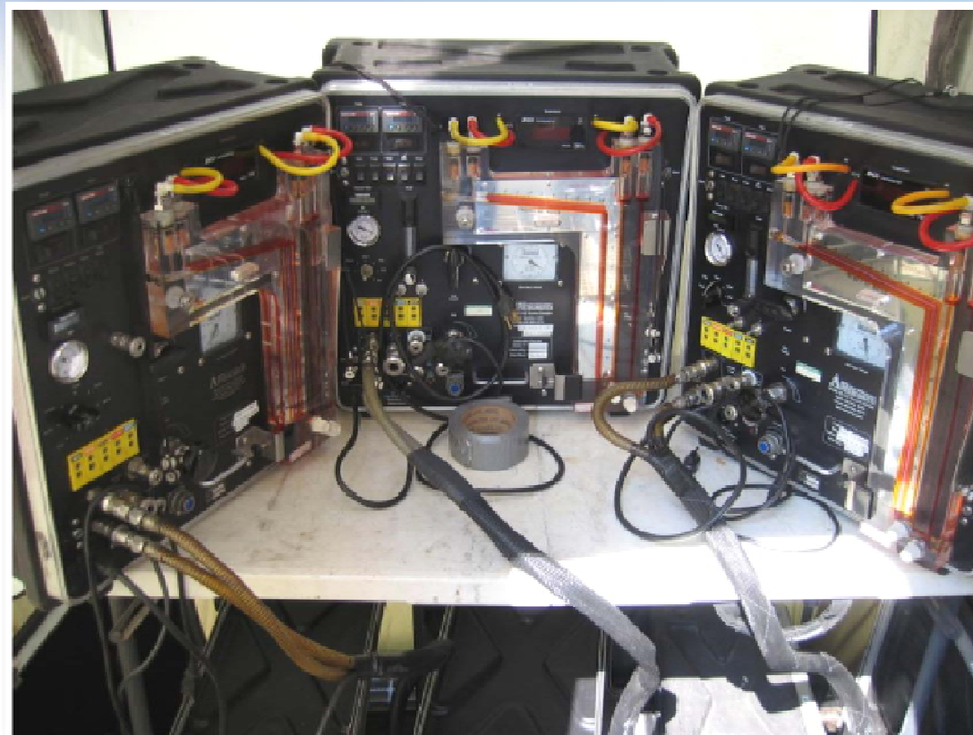
Flue Gas Pressure Drop (Manometers)
